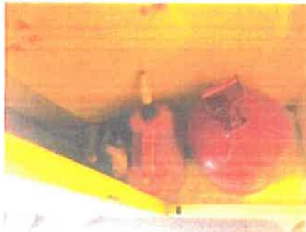
Photograph 11. View of the flammable storage cabinet containing small portable fuel containers.
