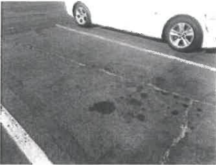
Photograph 13. View of surficial staining on asphalt located in the parking lot area on the subject property.
